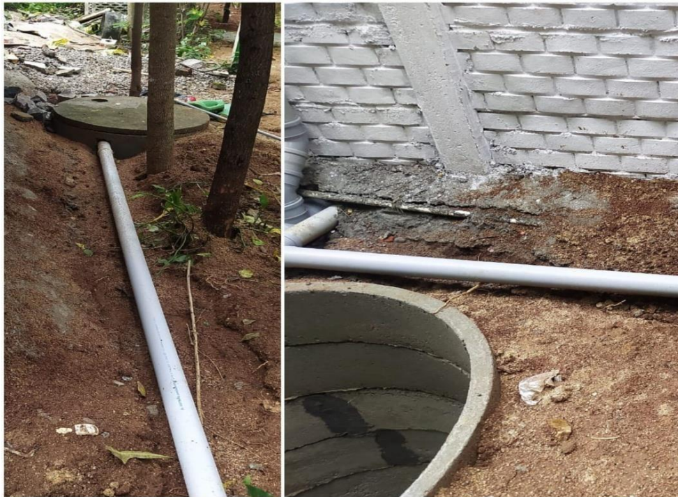
Water soaking pit for used water
