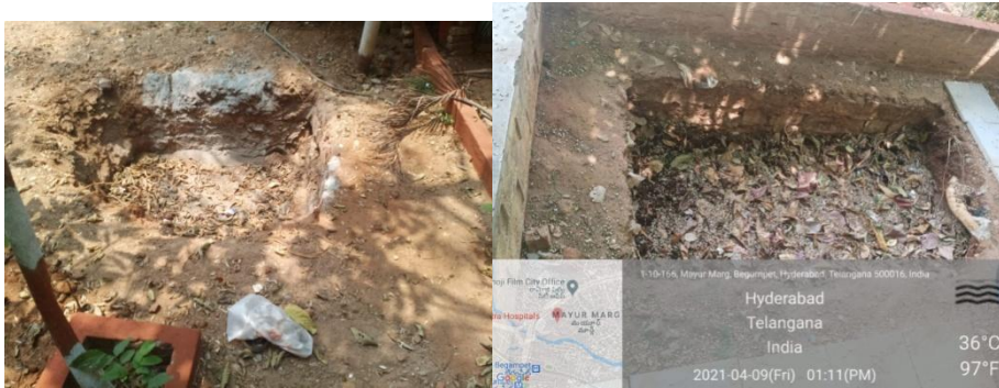
RAIN WATER HARVESTING PIT
