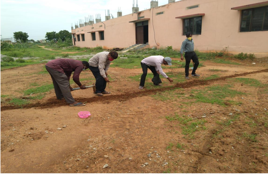
Chanalising waste water
