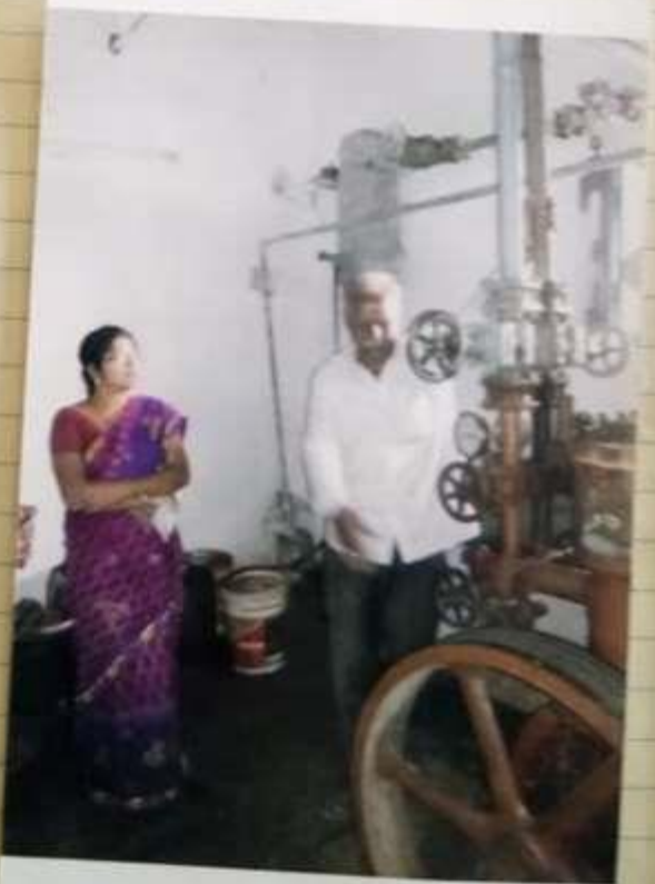
Machinery used in ice formation process by supply of NH_3
