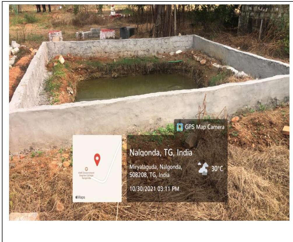
Rain water harvesting pit
