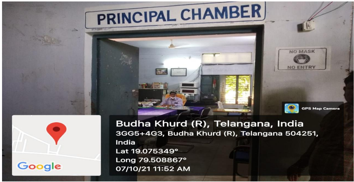
LED bulbs In Principal Chamber
