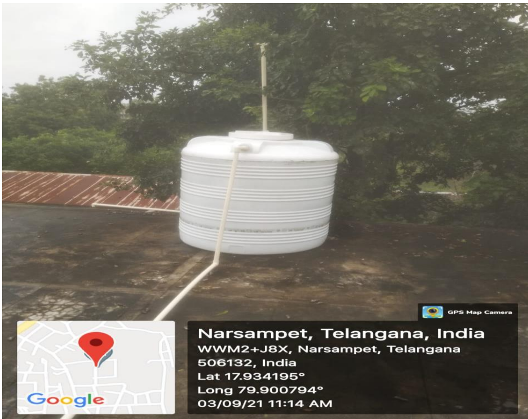
Newly Installed Over Head Tank on the Principals Chamber Roof for the water supply to the Principals Office & Haritha Haram Plants.
