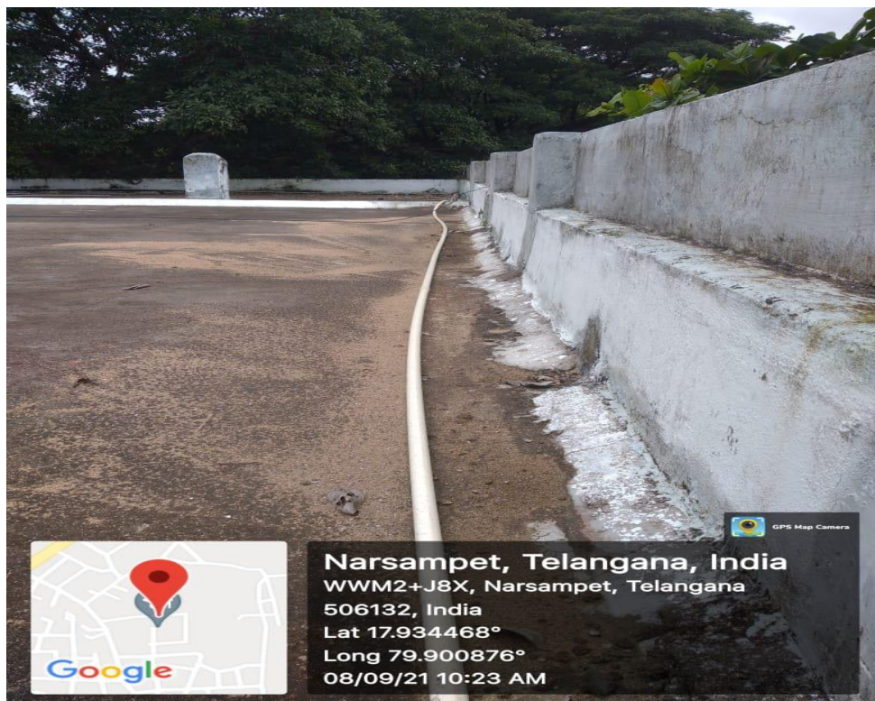
Pipe line System for the Supply of Water from the Over Head Tanks to Botany, Zoology and Chemistry Laboratories, R.O. Plant & Washrooms
