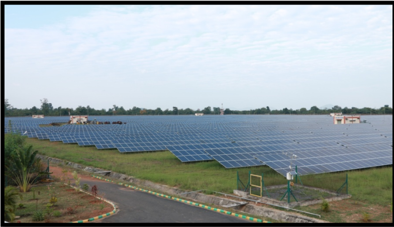
12 MWp Solar Power Plant
