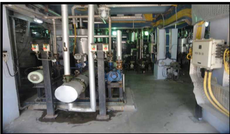
Oxygen -18 enriched water production facility
