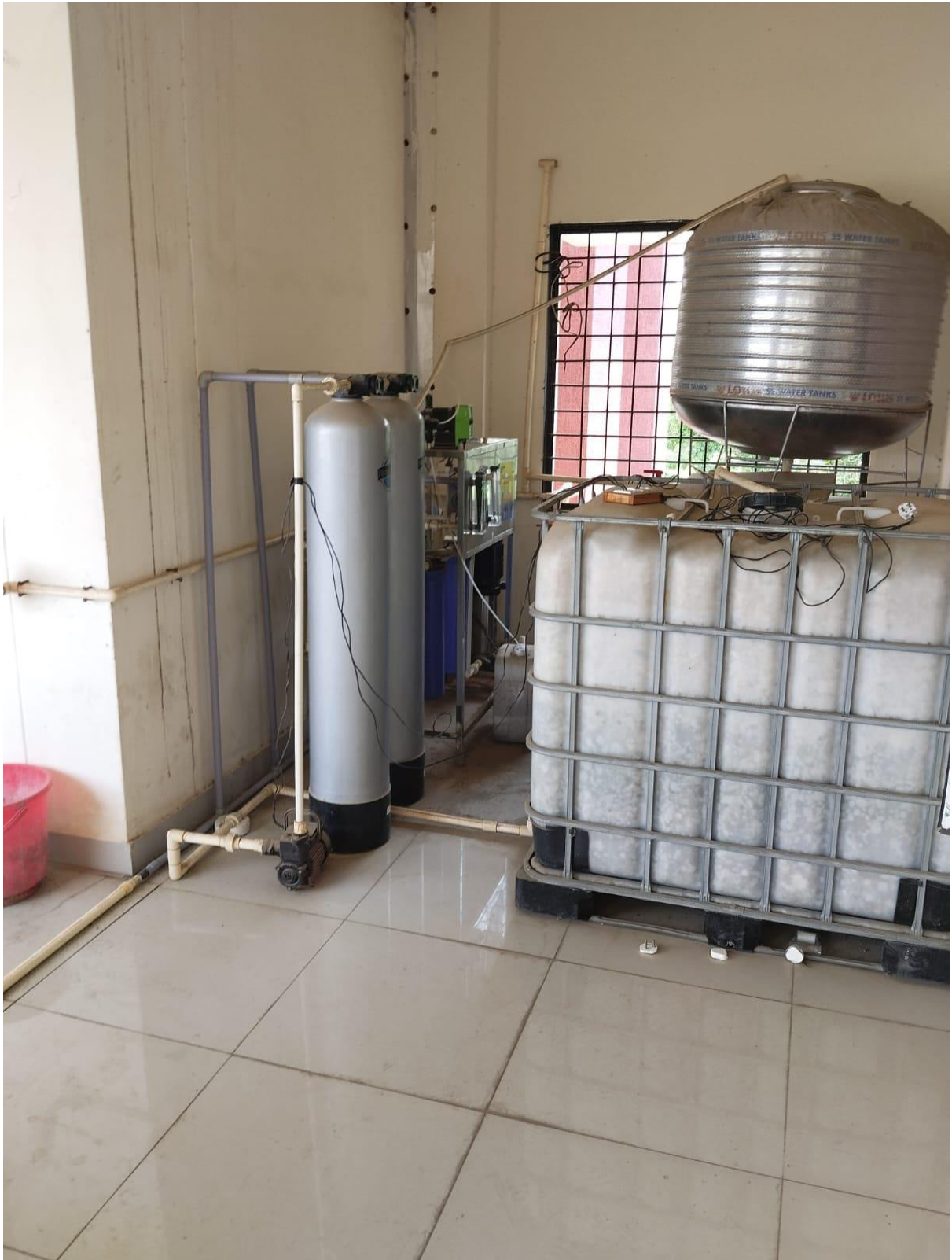
RO WATER PLANT
