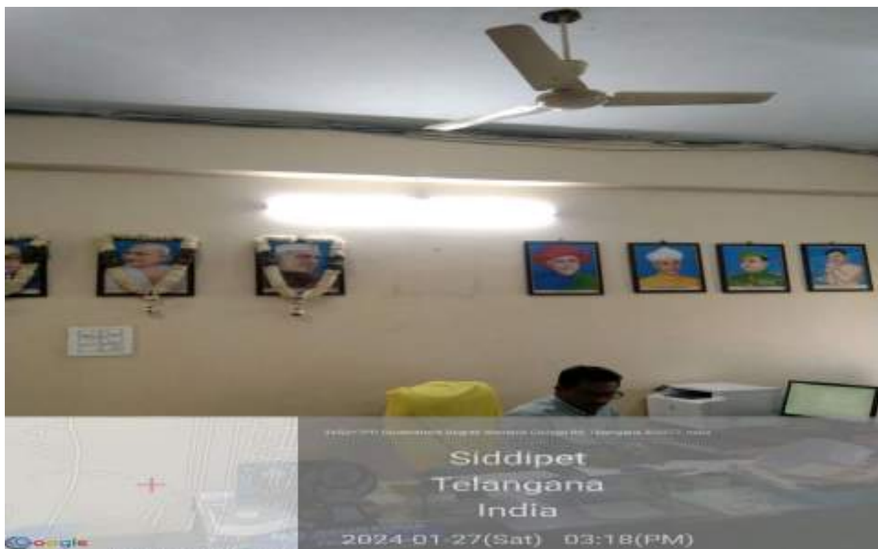
LED tube light in principal chamber
