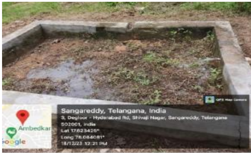
RO waste water into the water harvesting pit
