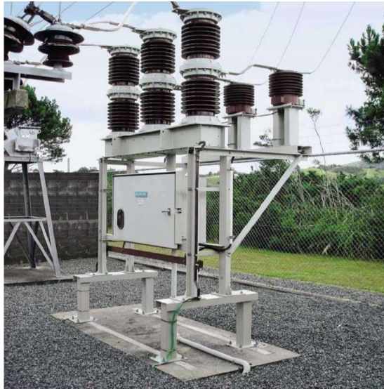
FIG: CIRCUIT BREAKER
