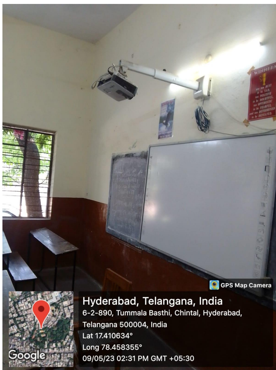
ICT facility in in Room No .4
