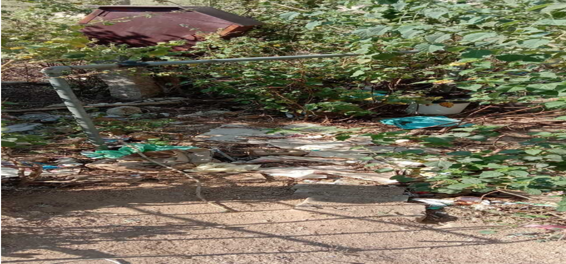
Bore well is used in institute for water needs
