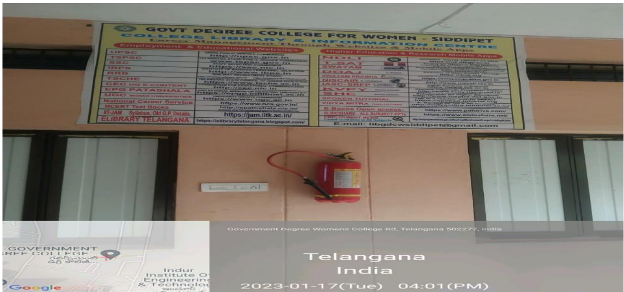
Fire extinguishers have been installed outside the library
