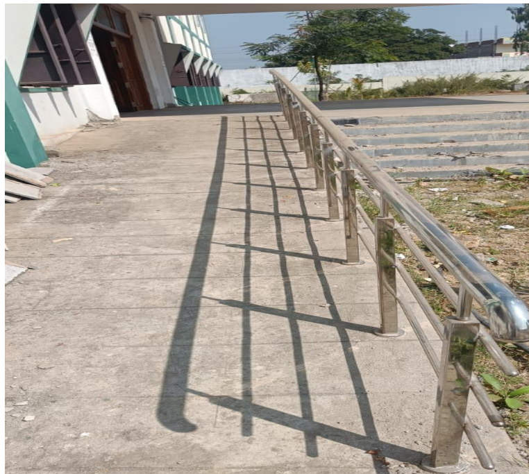
Ramp available for Divyang Jan
