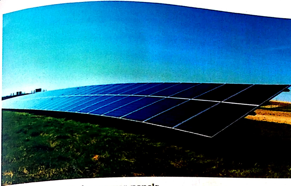
Fig. 3: Solar power panels
