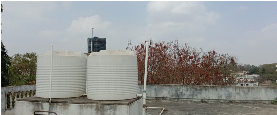
Water tanks are allocated in campus
