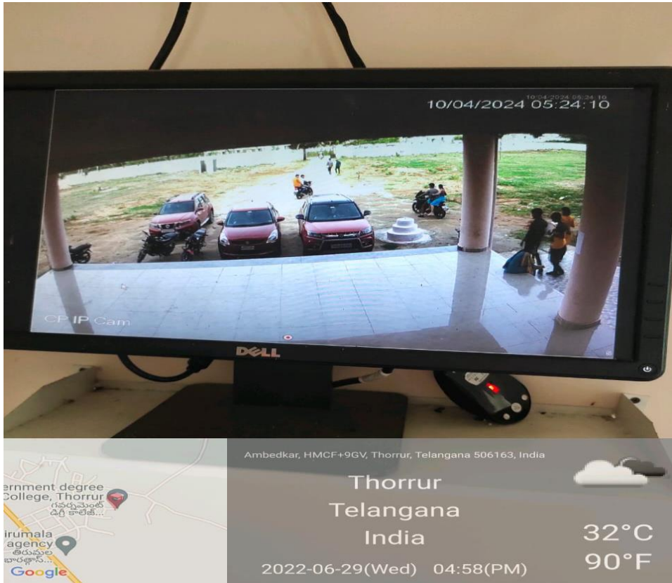
CC CAMERAS at ENTRANCE
