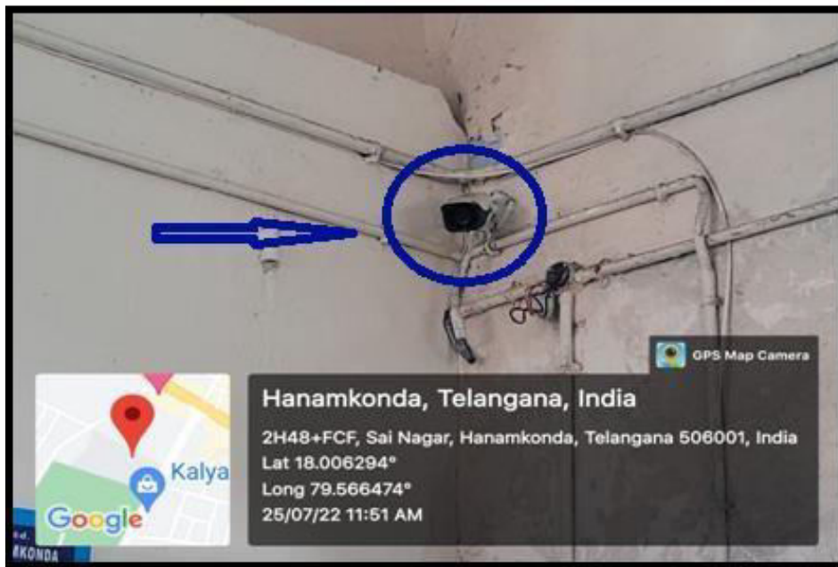
CC Camera in front of the Office Room
