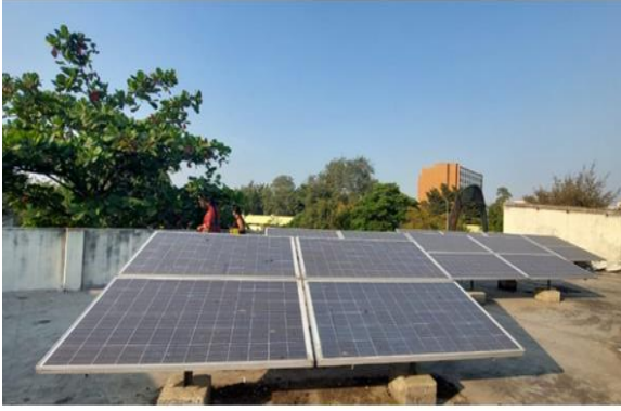
Solar Power Plant
