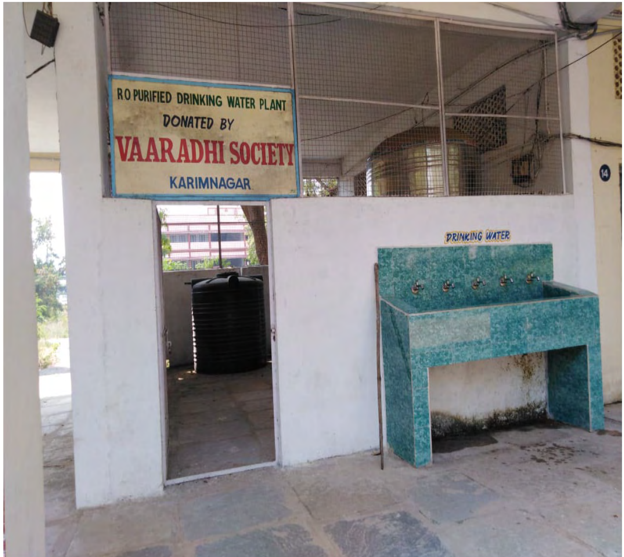
R.O. Water Plant
