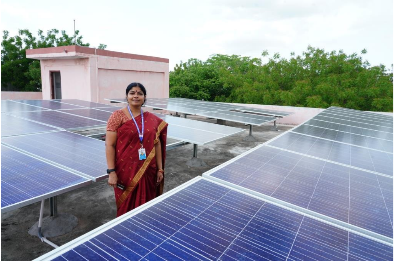
Solar Power Plant
