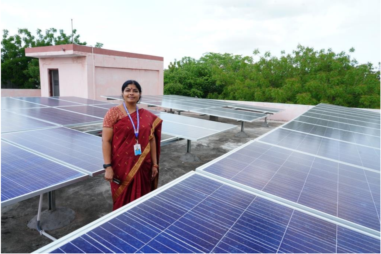
Solar Power Plant
