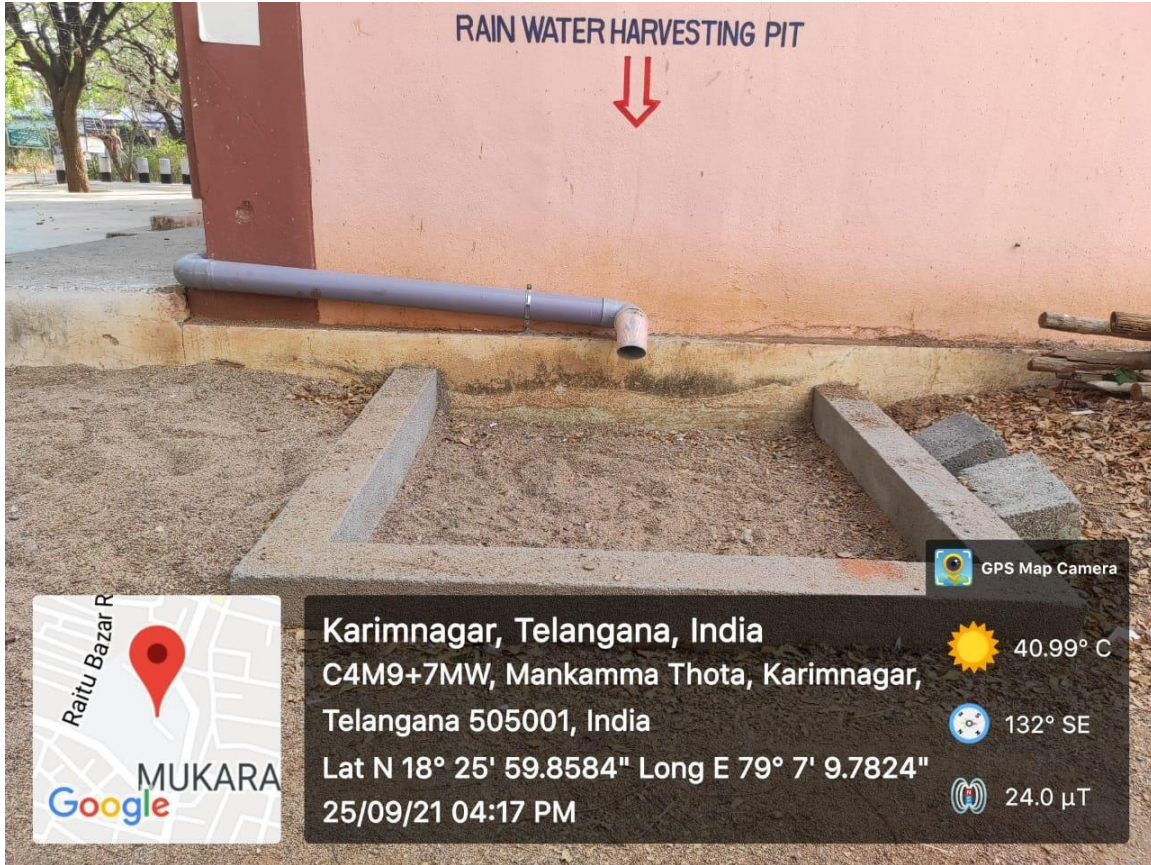
Rain water harvesting pit 01
