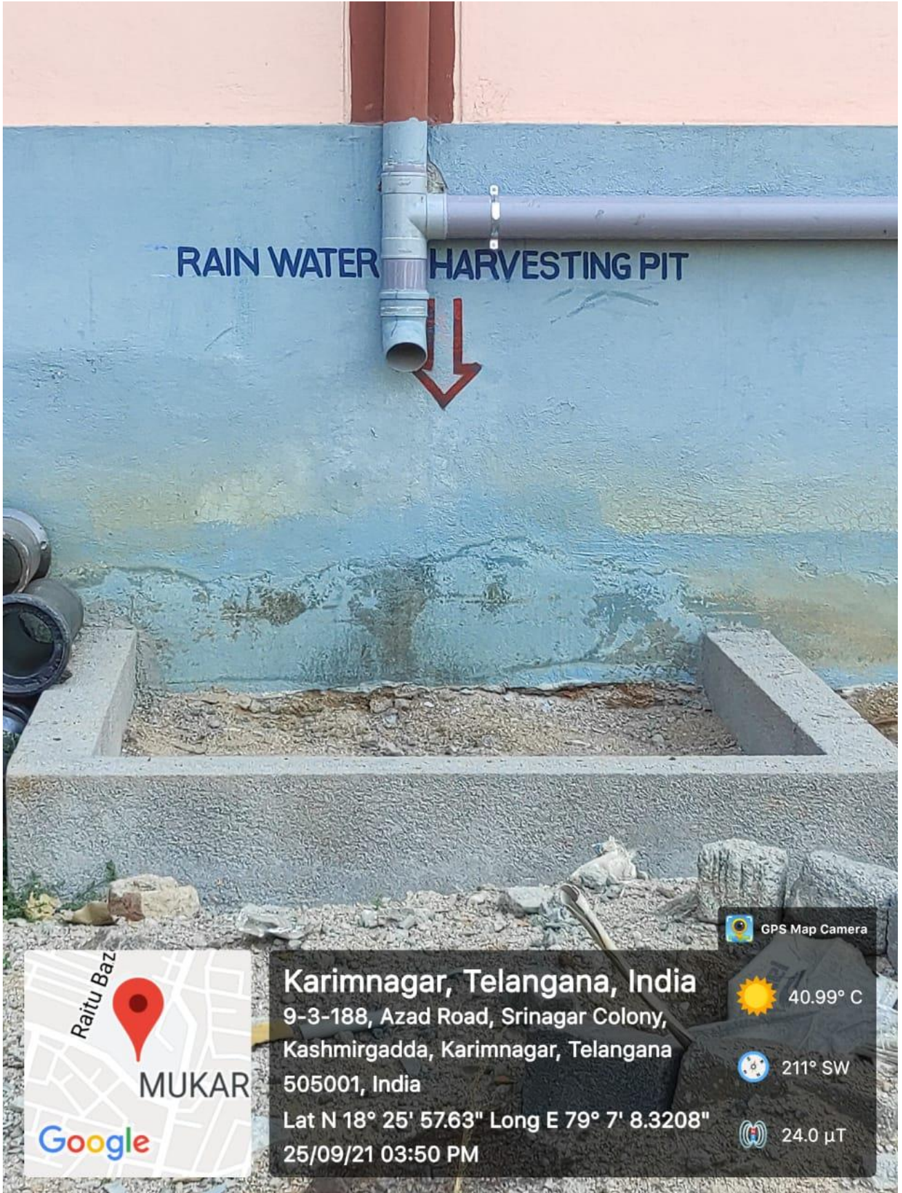
Rain Water Harvesting Pit at CHEMISTRY BLOCK
