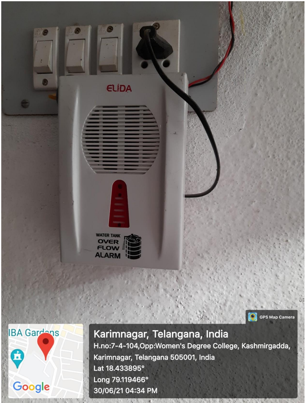
Water overflow alarm for Energy conservation
