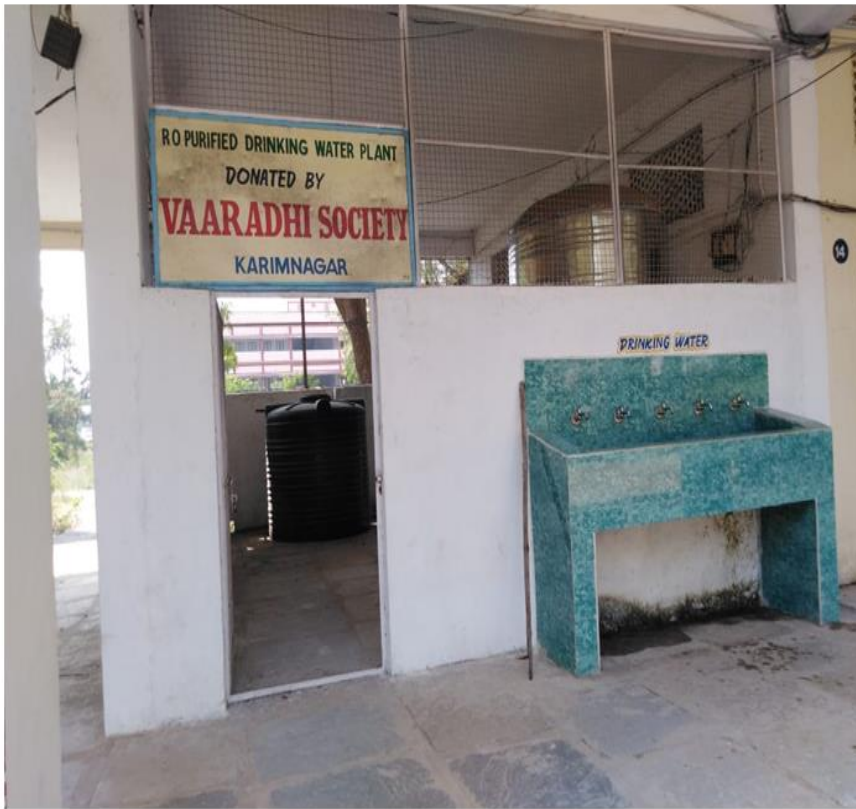
R.O. water plant
